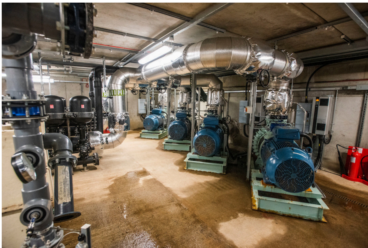
Equipment beneath the River Clyde at Queens Quay District Heating Network
