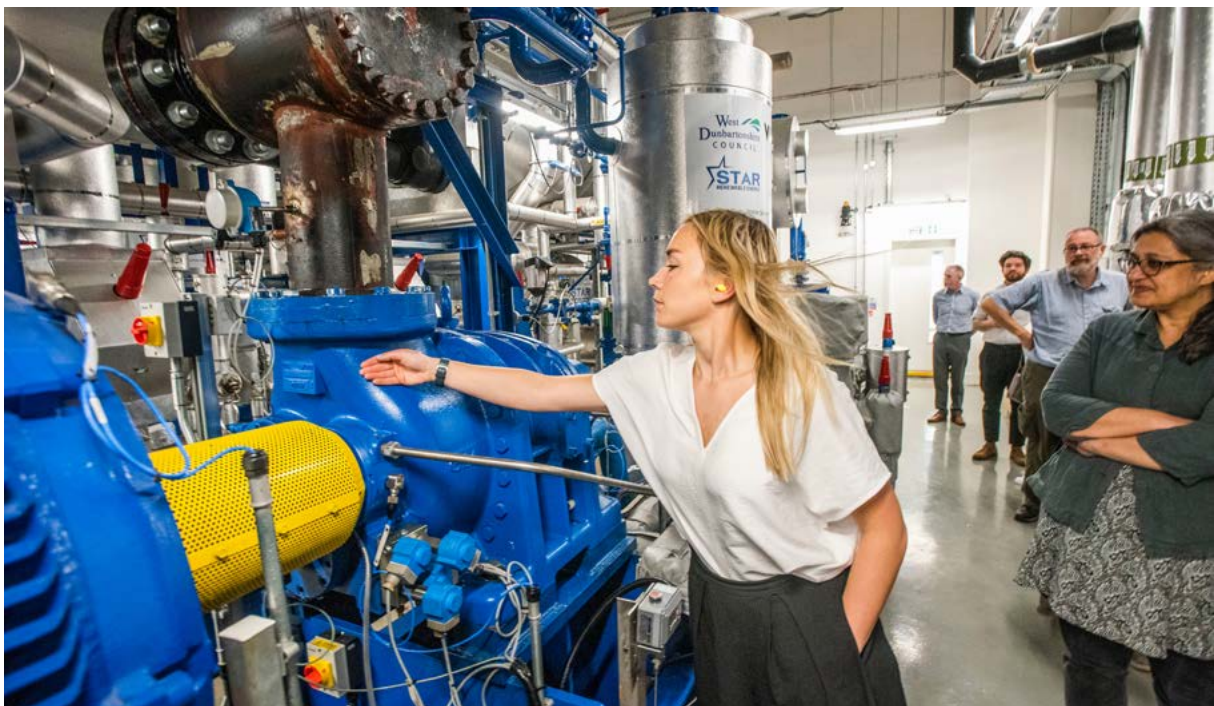
Commissioners tour the pump system at Queens Quay Energy Centre, Clydebank
